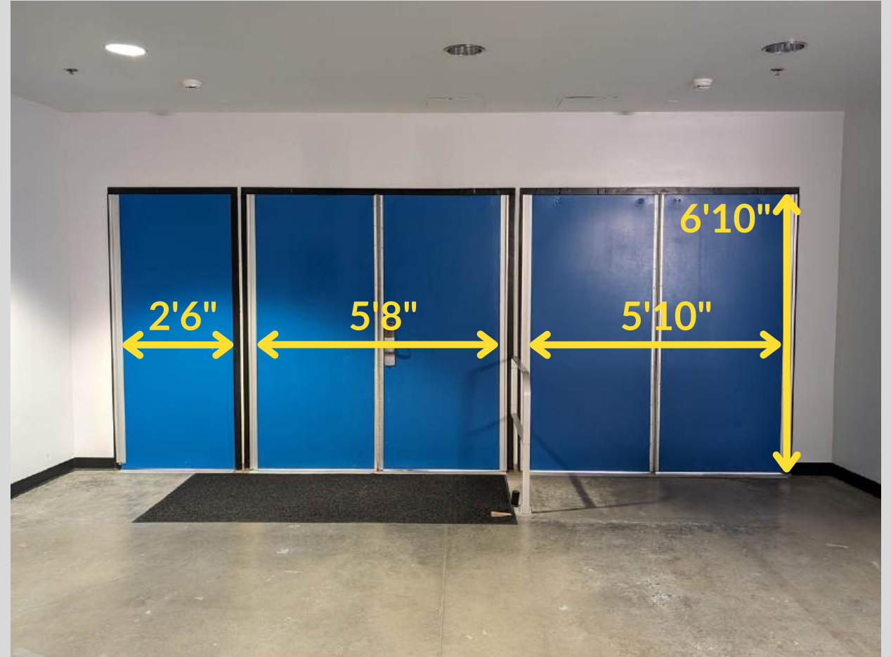
Entry Doors (1 single door; 2 double doors)
